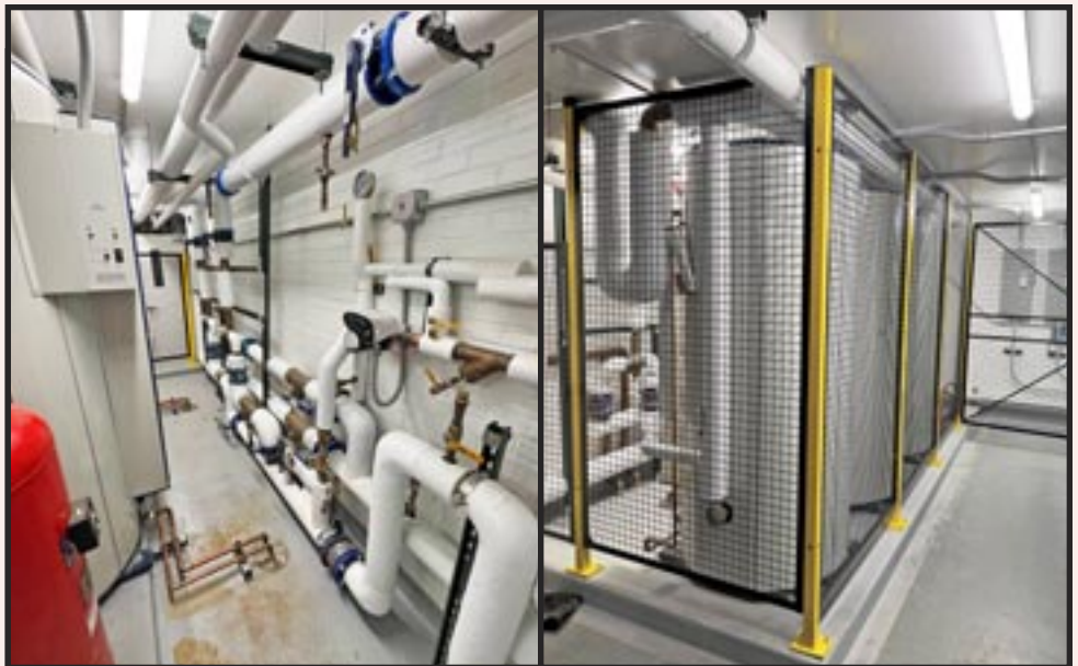
Shown in both photos is an electric domestic water heating plant.
