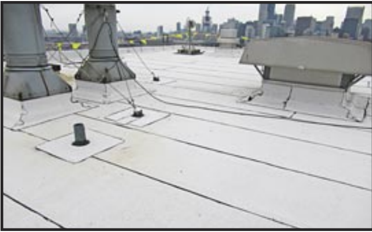
➤ Roof replacement and repairs are among the most common projects for Chicago area buildings.
