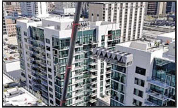
➤ Replacement of mechanical equipment including chillers as shown in this photo are common projects for Chicago high rise buildings.
