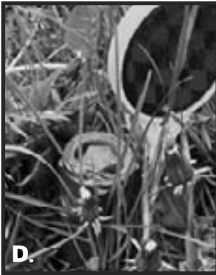
D. Damaged B-Box
